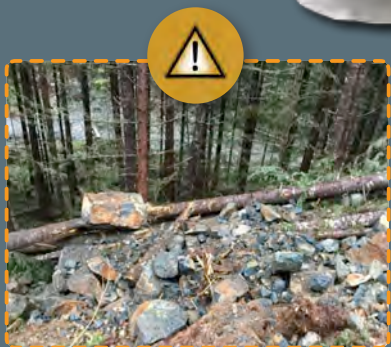
Logs and debris out of reach of machines
